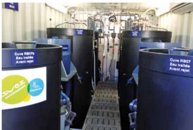
Advanced treatment tests of the Université de Limoges at the cooperating SIPIBEL site (F)
